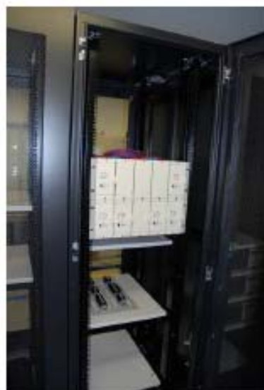
Fig.8. External view of multiple SiC-SIT circuit breakers installed in a communication system rack.
