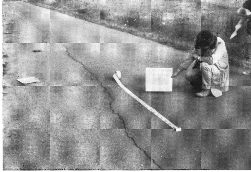
Photo. 1 The Crack of Side Road
