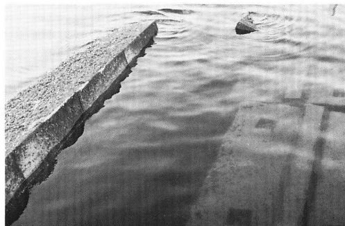
Fig. 6 Photo of damaged breakwater
