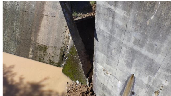
(b) leakage positions
