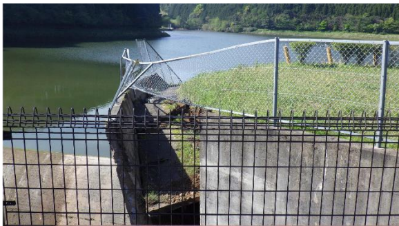
(a) Water diversion equipment damaged
